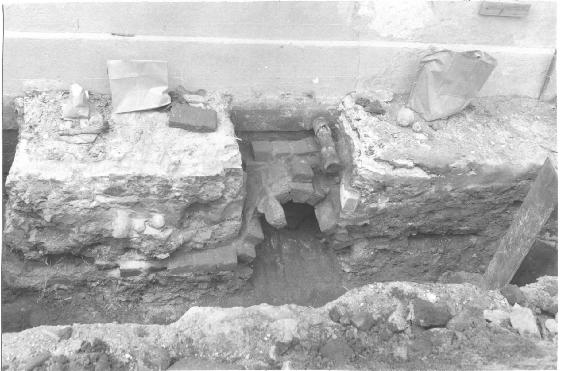
Figure 26. Photograph of the nineteenth century brick drain along the east wall of the Exchange Building in Section V. Note the iron drain pipe above it which goes into the wall.
